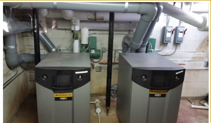
Above: New high efficient boilers in the boiler room.
